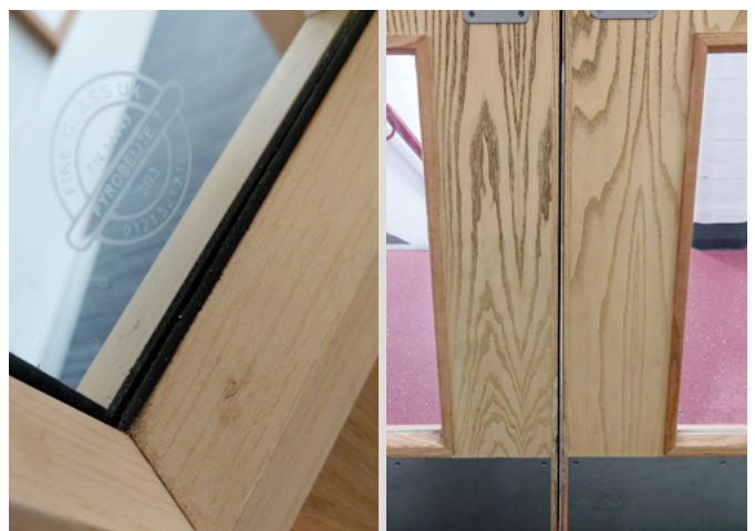
Lee had concerns about whether the fire doors in the school were compliant
