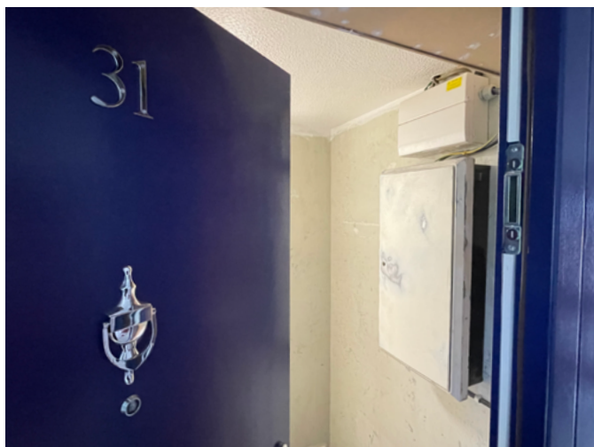
Remedial work was needed on electrical wires within the flat before the new doorset could be installed.
