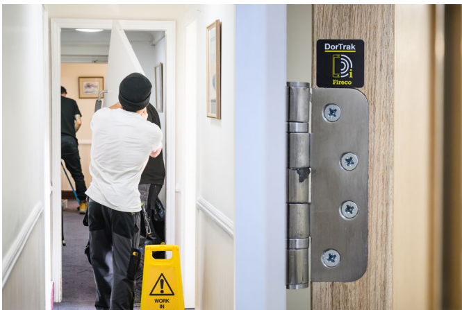
As part of our inspection service, fire doors are fitted with DorTrak tags to allow quick access to their service history.
